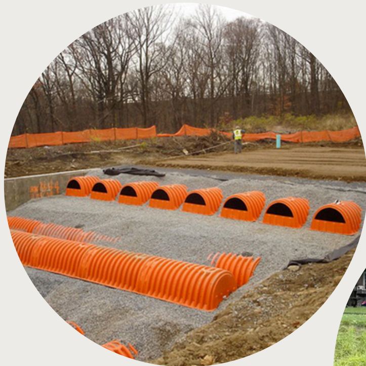
underground retention basins
